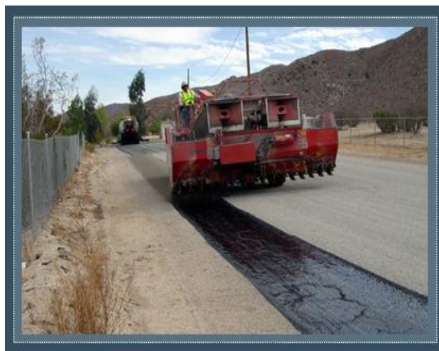
Figure 41: Fog Seal Poor Practice (NHI PPTCG 2007)
