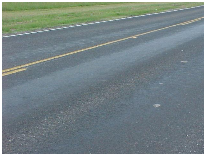
Figure 31: Bleeding Chip Seal (Webb 2010)
